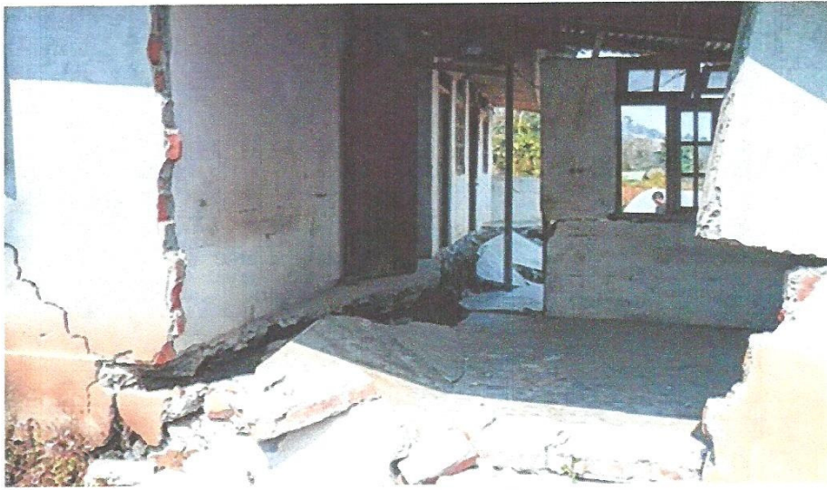
A wall of a house in Karthok village near the airport construction site that has almost collapsed
